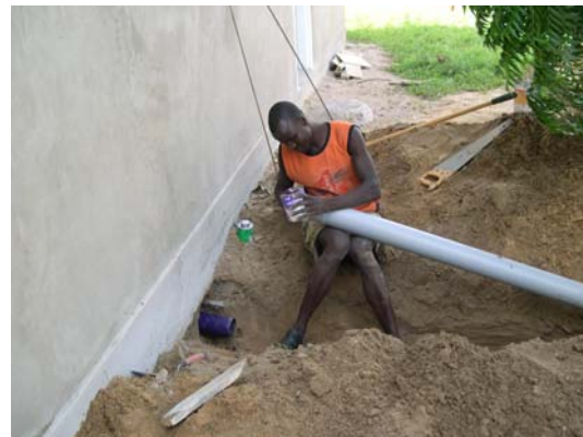
Chadian worker on CEF crew is connecting pediatric ward plumbing system to new septic tank out back.
