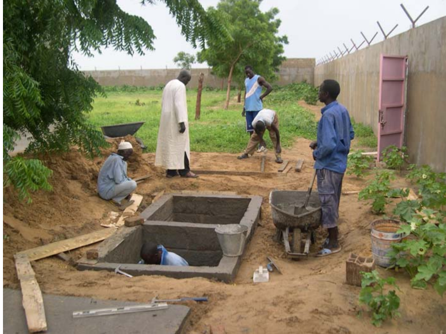
CEF Chadian crews putting the finishing touches on the fifth on site septic system. Next the crew will enlarge the septic system capacity for the hospital clinic building, and install a new drywell system. As the funding is received, a new, larger water tower will need to be erected for increased water capacity and pressure.
