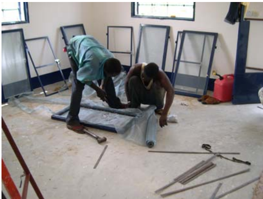
Workers above are installing the windows and window screens in the second doctor's house.
